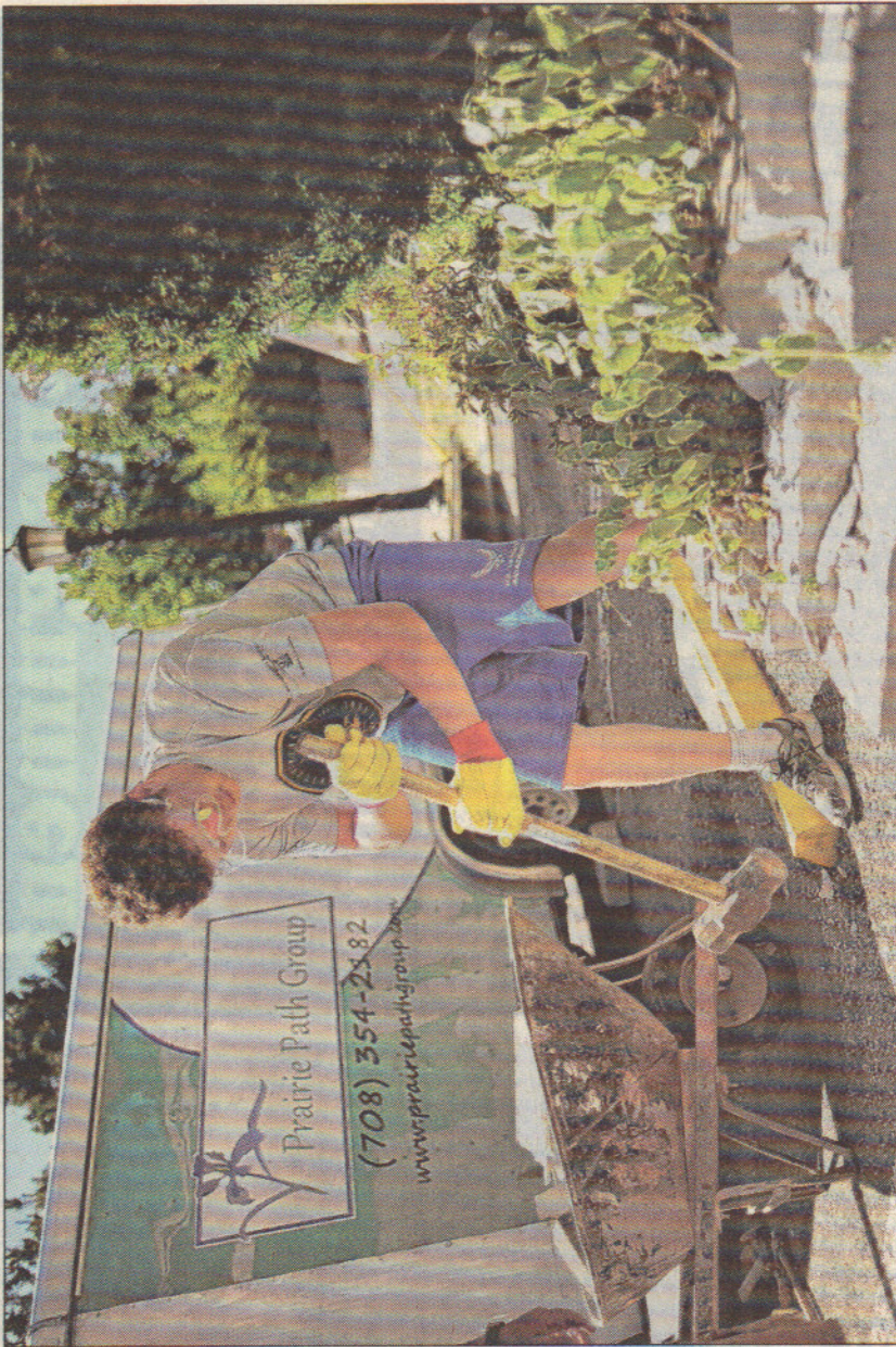
Aaron Brown uses a sledgehammer to demolish a brick wall for his Eagle Scout project at the Hinsdale Humane Society. | ROB HART-SUN-TIMES MEDIA
